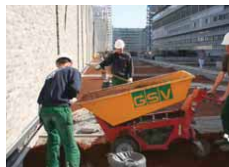
Motorized wheelbarrows makes it easier to transport the substrate on the roof.
