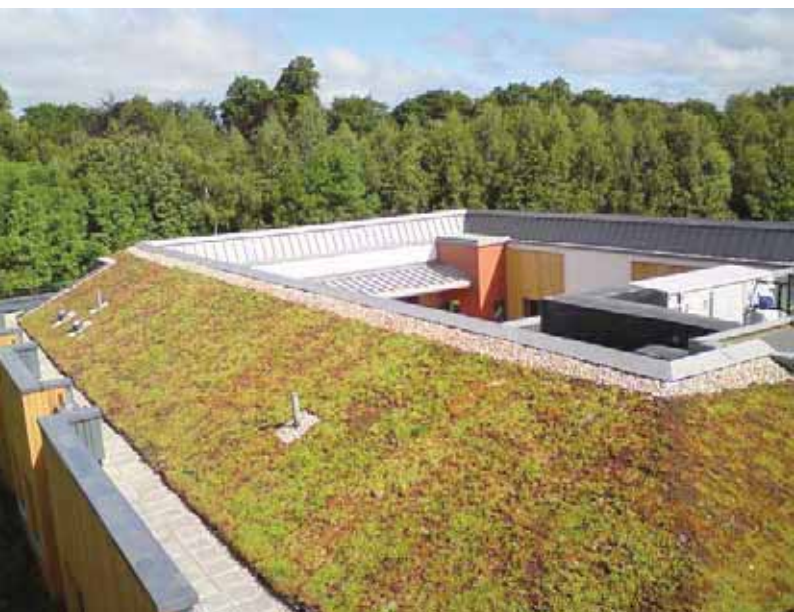
Extensive Green Roof, Harperbury, Copyright Alumasc
